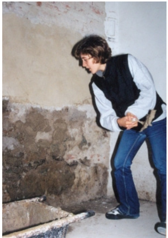
Fig. 5. Traditional plastering: training consisted of theoretical part (technologies, materials and tools), as well as practical exercises of preparation of various kinds of plaster mixtures on the base of lime, and wall plastering.
